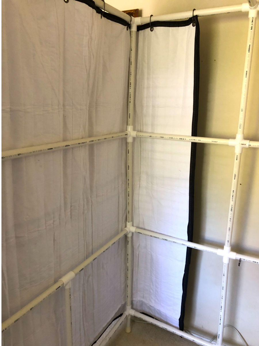
Booth corner detail with first blanket attached. I start at the left corner and work to the back. This is the Producer's Choice Sound blanket and the shower curtain rings from the parts list.
